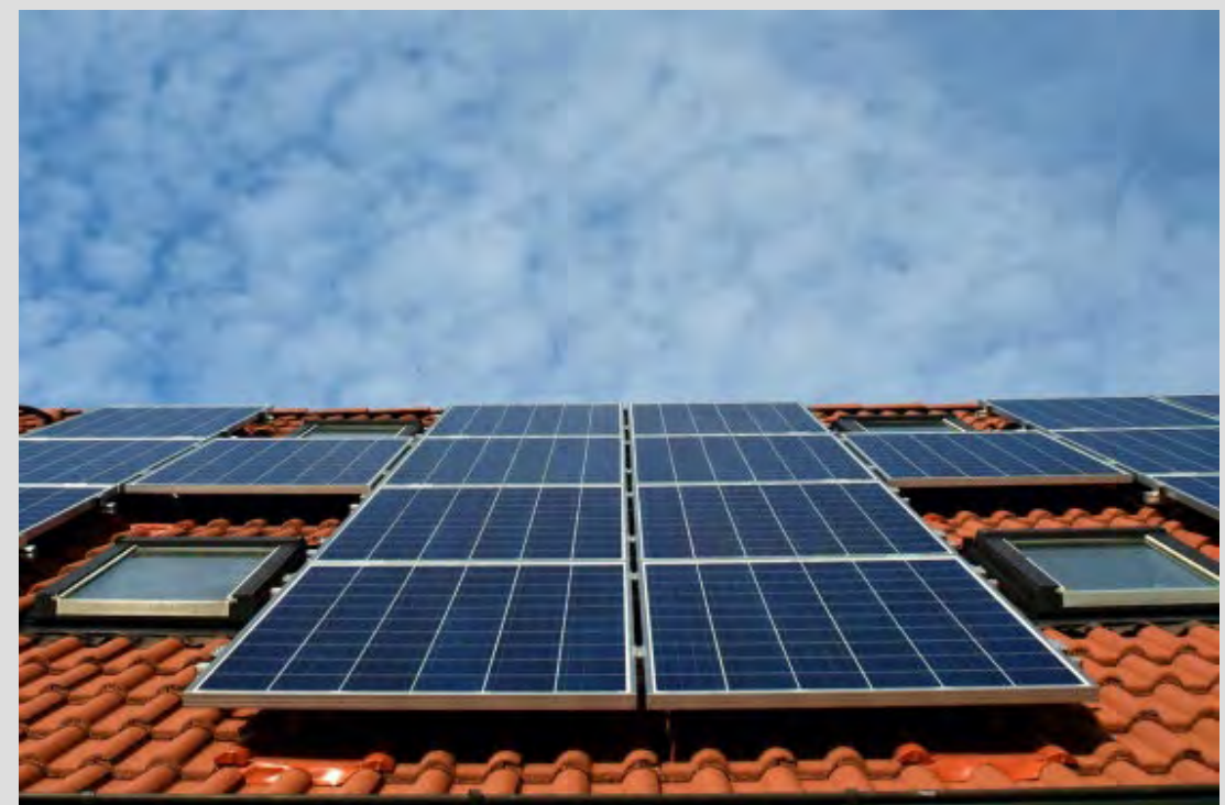
Figure 23: Solar Panels photo credit: Worcestershire County Council
