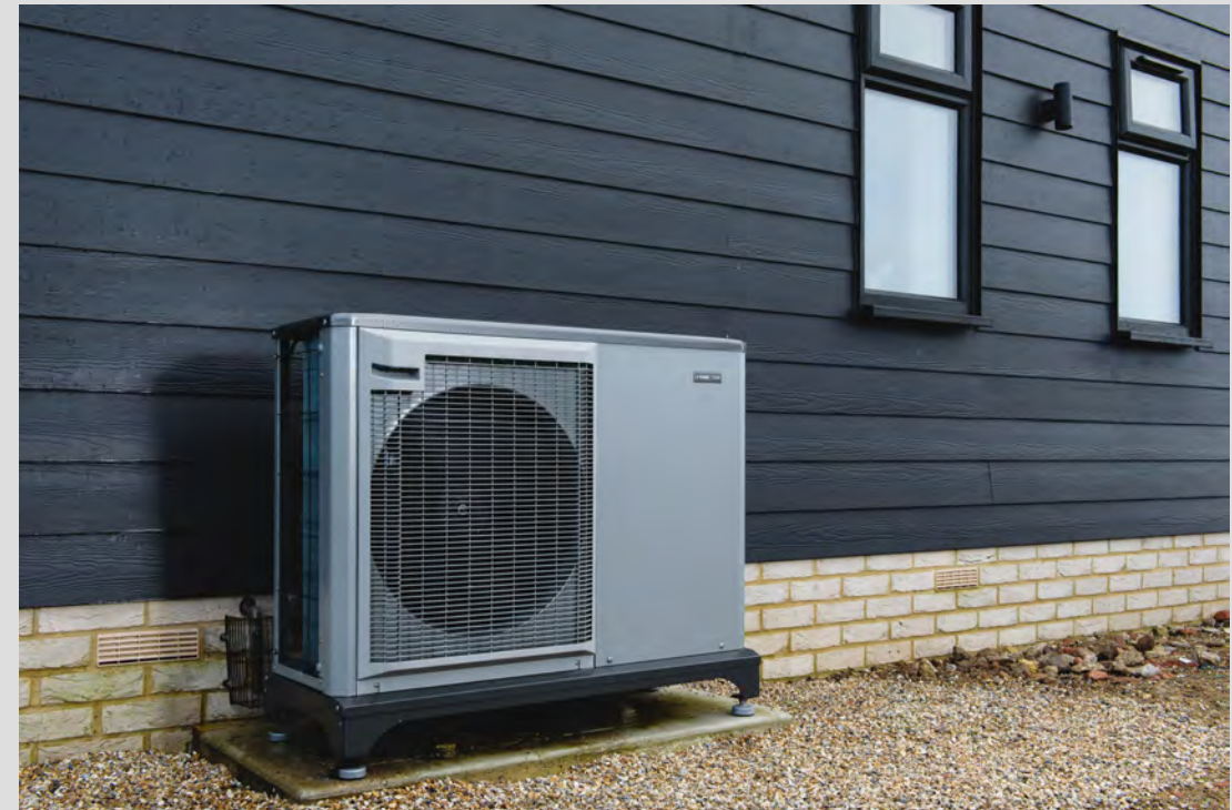
Figure 22: Example of an Air Source Heat Pump: Photo credit Nu-Heat
